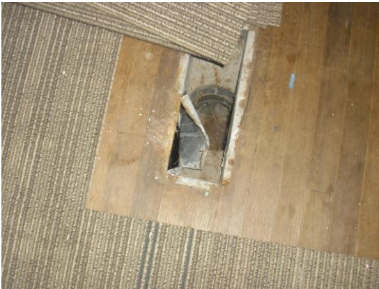
Floor 1 Room 1 Unwrapped Register
