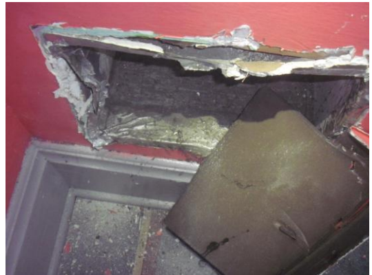
Floor 2 Room 3 Unwrapped Register
