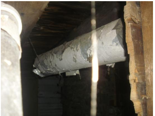
Basement Pipe with Wrap
