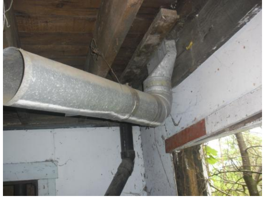
Basement Room 2 ducts no wrap
