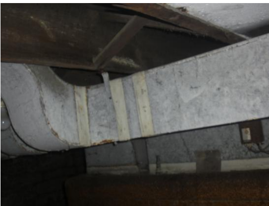
Basement Ducts with Wrap
