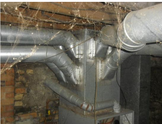
Ducts no Wrap
