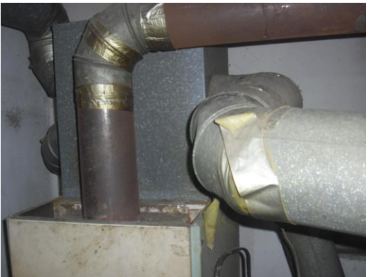
Ducts on Furnace No Wrap
