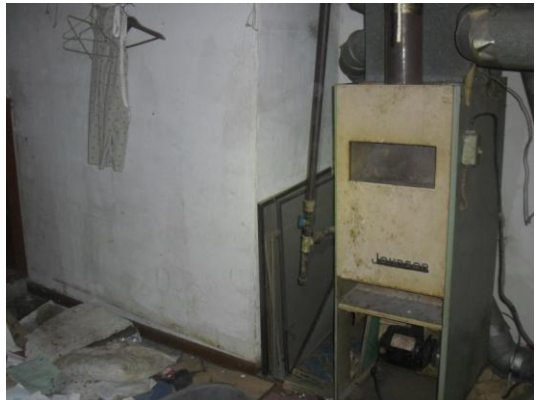
Floor 1 Room 4 Furnace
