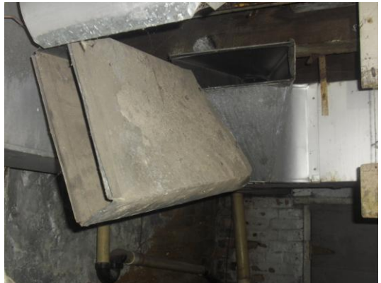
Basement Ducts No Wrap
