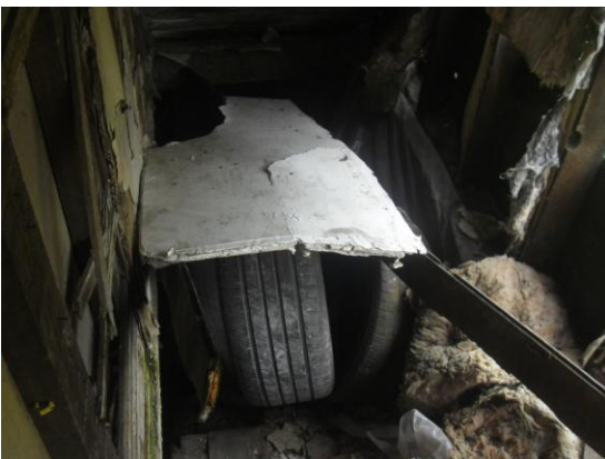
Barricaded Basement Stairs
