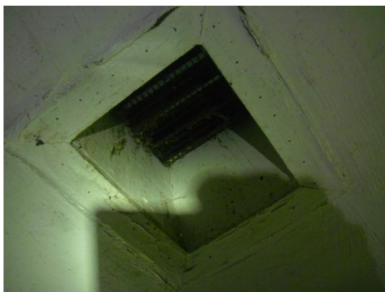
Floor 1 Room 3 Heat Pass Through
