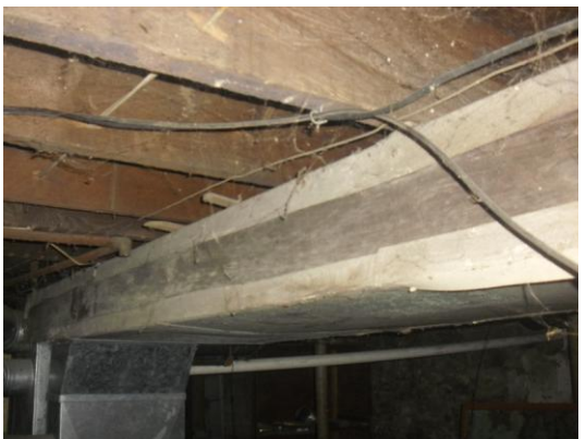
Basement Ducts with Wrap
