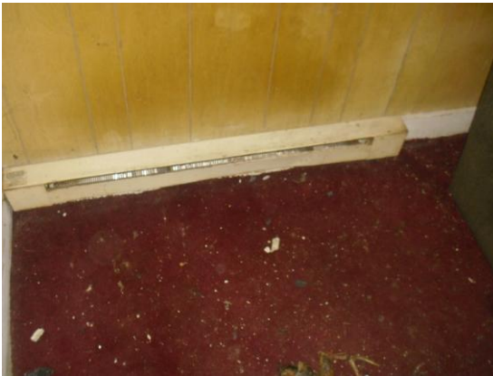
Floor 1 Room 1 Radiator
