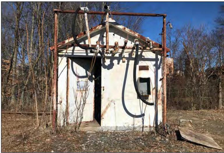
Photo 5: View of pump house to west of garage. View is facing to the north.
